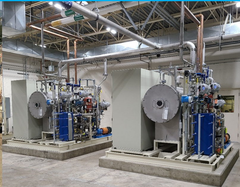
Duff Water Treatment Plant Ozone Generator
